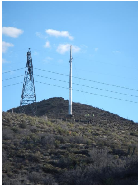
Photo 6: Steel pole 75 was erected during this reporting period. Work activities were observed being completed within the approved work limits as required in MM-BIO-1a.
