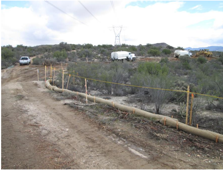
Photo 5: Water trucks are utilized during clearing and grading activities associated with steel pole pad sites for the overhead alignment in accordance with MM-BIO-4a.
