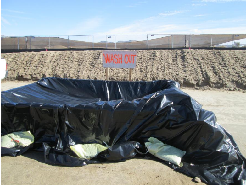
Photo 1: A concrete washout is utilized at the Boulevard Substation Rebuild site during concrete pours associated with substation foundations in accordance with MM-HYD-1 and the SWPPP.
