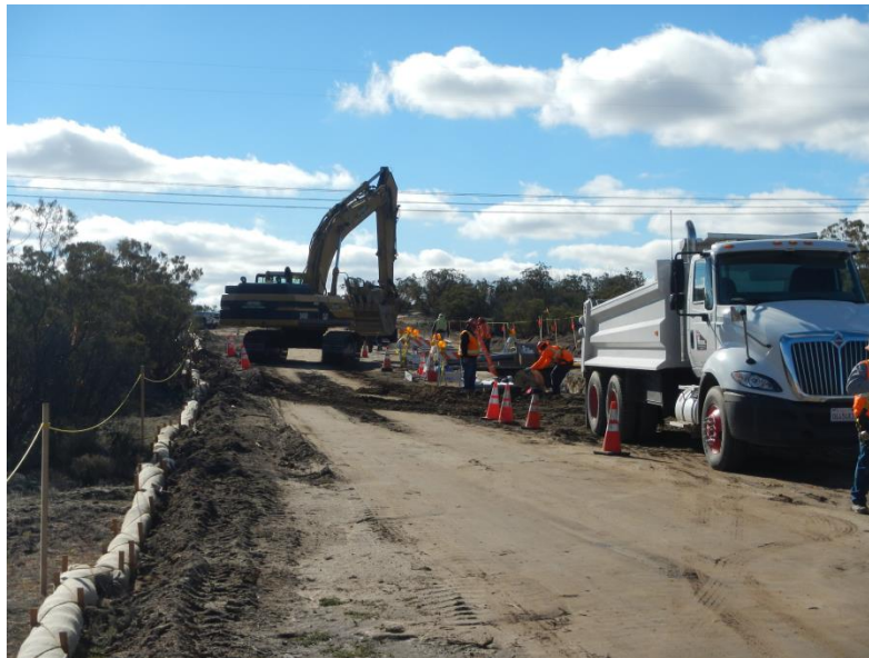
Photo 4: Yellow ropes are utilized to delineate the approved work limits during construction activities associated with the underground alignment in accordance with MM-BIO-1a. BMPs consisting of straw wattles are also placed along the work limits in accordance with MM-HYD-1 and the SWPPP.
