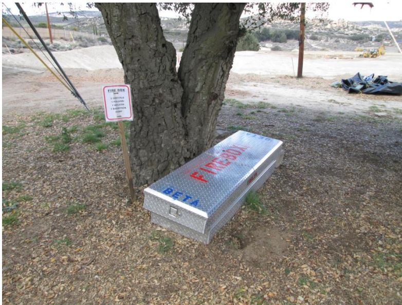
Photo 2: A Fire Box containing fire equipment is maintained onsite at the Boulevard Substation Rebuild Site in accordance with the Construction Fire Prevention Plan (Mitigation Measure FF-1).
